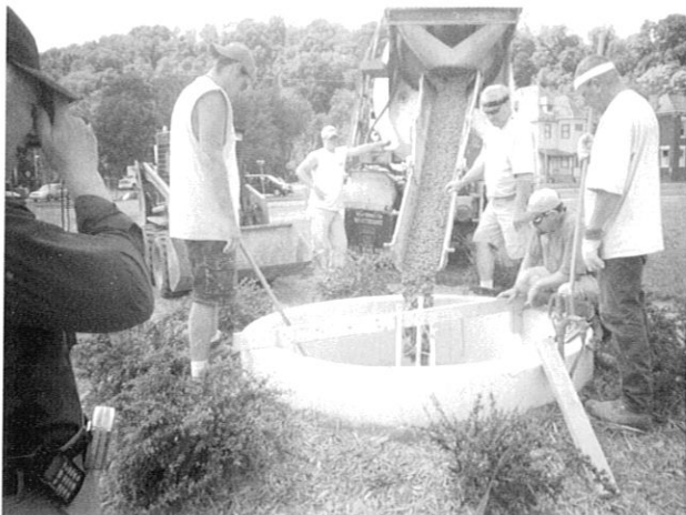
Dick Boulton Construction donates time and resources to help build Restoration Park (near the Sixth Street Bridge). The Park opens in the fall of 2003. (Photo by Kate Hagemeyer)
