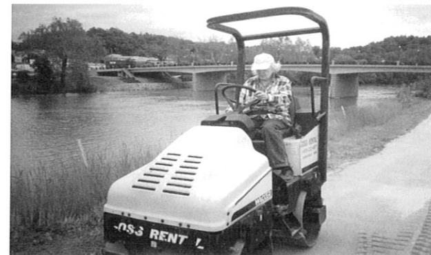
Kate Hagemeyer paves walkways in Restoration Park, with the generous donation of equipment by Goss Rental. (Photo by Bart Hagemeyer)
